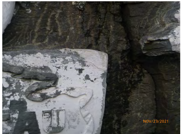
47-12 Stone_Repair Patch Failed 2021-1
