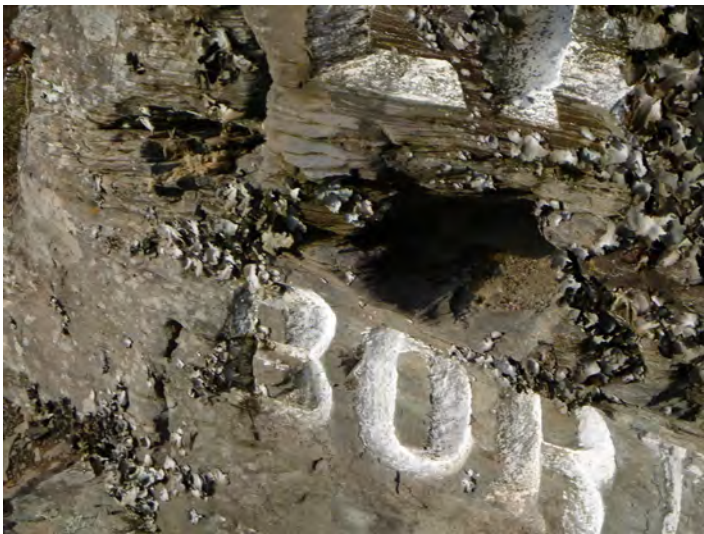
32-17 Stone_Crack Single unit 2021-2
