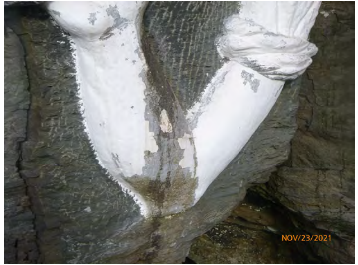
50-8 Stone_Coating Coating Failed 2021-2
