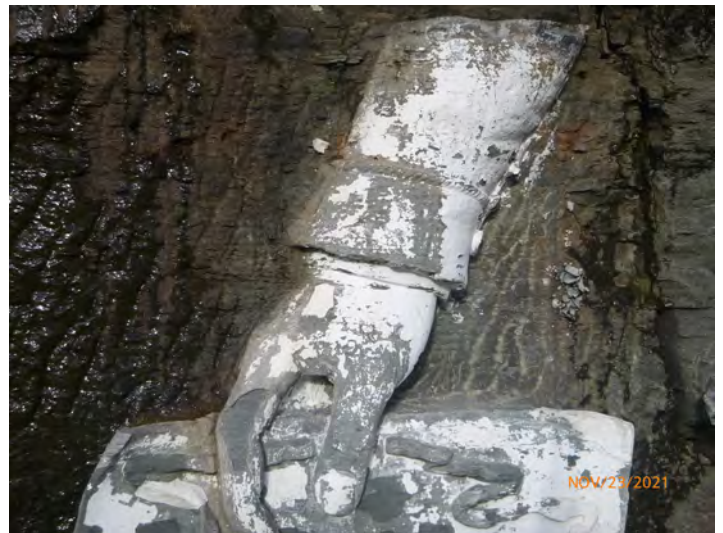
44-9 Stone_Coating Coating Failed 2021-2
