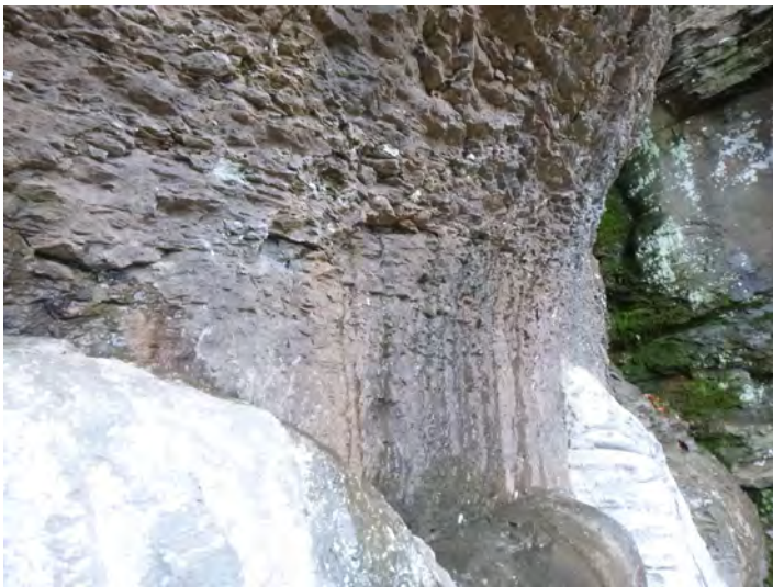
1-15 Stone_Note Photo-water seepage 2021-1
