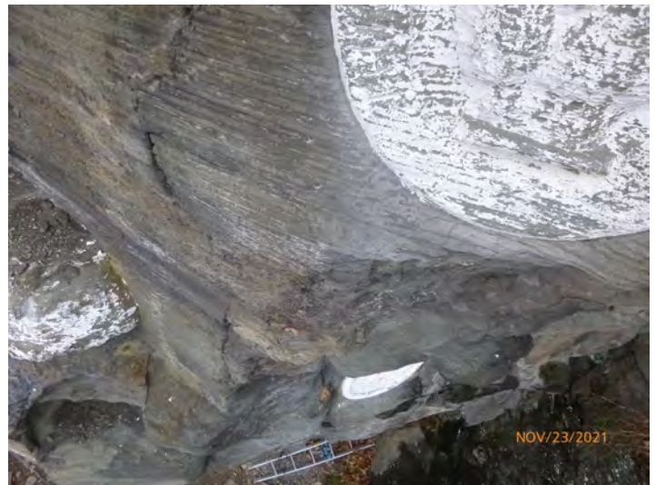
19-22 Stone_Crack Single unit 2021-3
