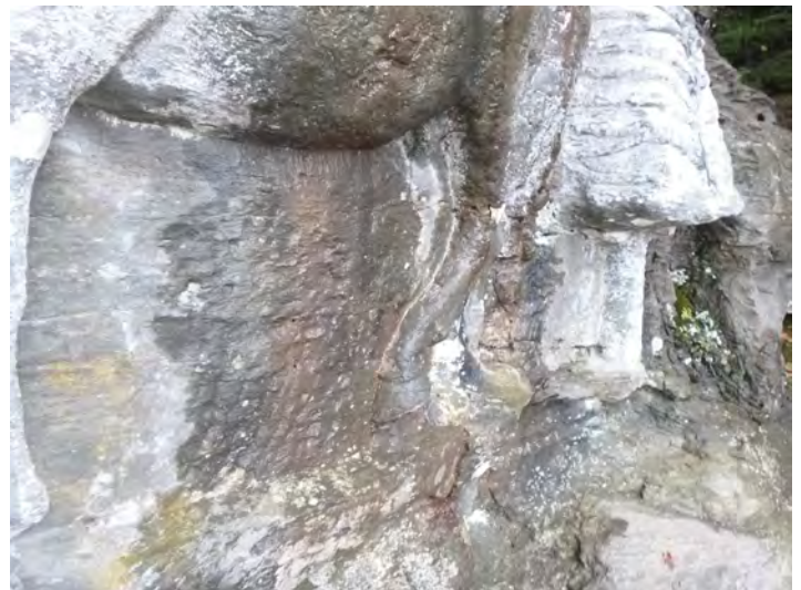
0-13 Stone_Note Photo-water seepage 2021-3
