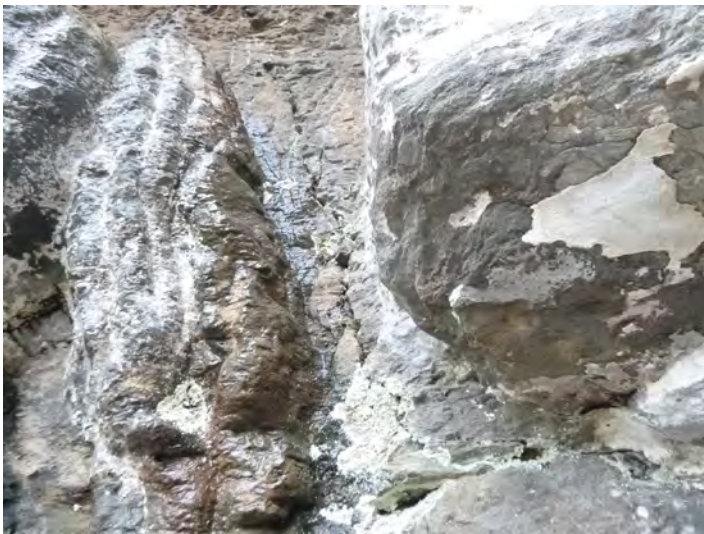
3-13 Stone_Crack System units 2021-2
