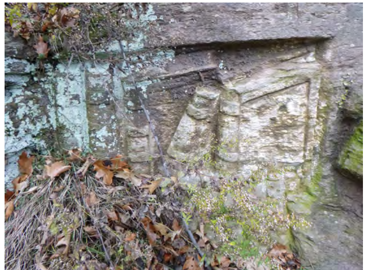
9-20 Stone_Coating Coating Failed 2021-1
