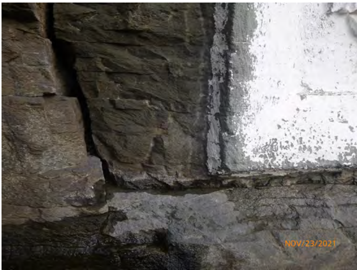
54-15 Stone_Crack Single unit 2021-4
