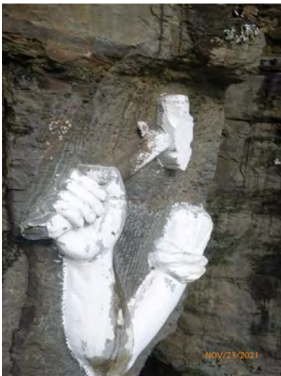
50-12 Stone_Note Photo-water seepage 2021-2
