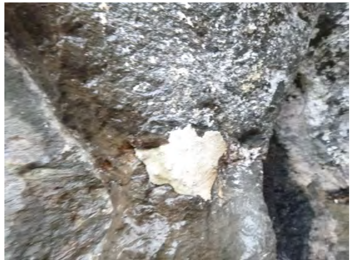
1-12 Stone_Repair Patch Failed 2021-1
