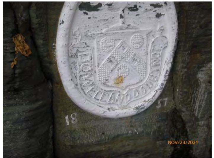
22-16 Stone_Coating Coating Failed 2021-2
