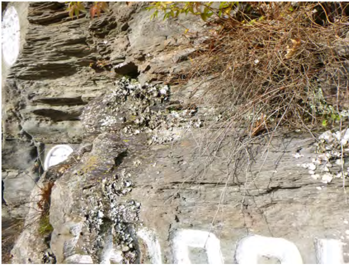
31-18 Stone_Note Photo- Water Seepage 2021-1
