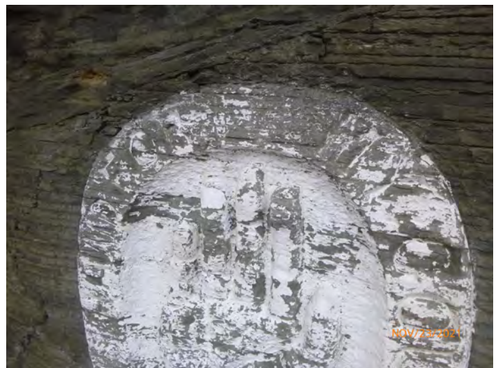
21-22 Stone_Coating Coating Failed 2021-1
