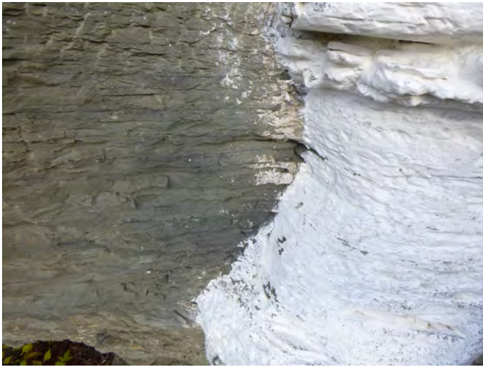
39-24 Stone_Crack Single unit 2021-1
