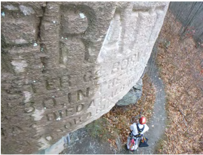
12-18 Stone_Coating Coating Failed 2021-2
