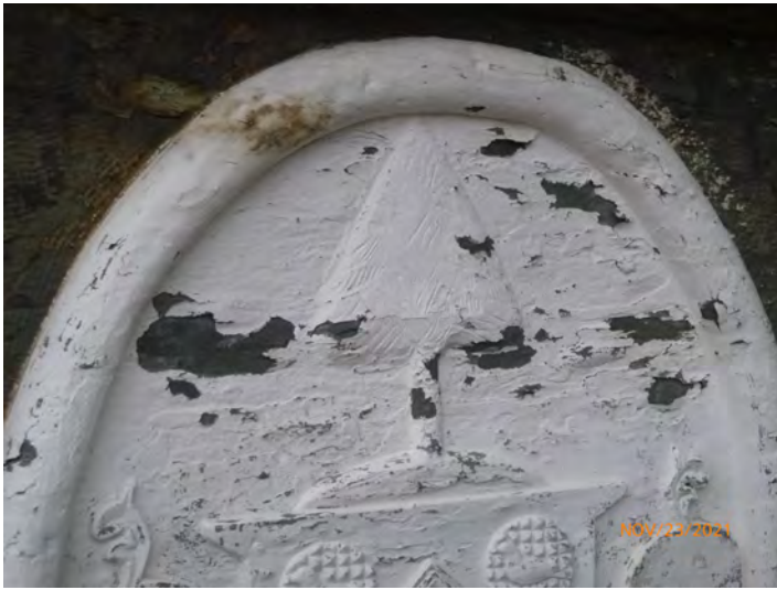
22-16 Stone_Coating Coating Failed 2021-3
