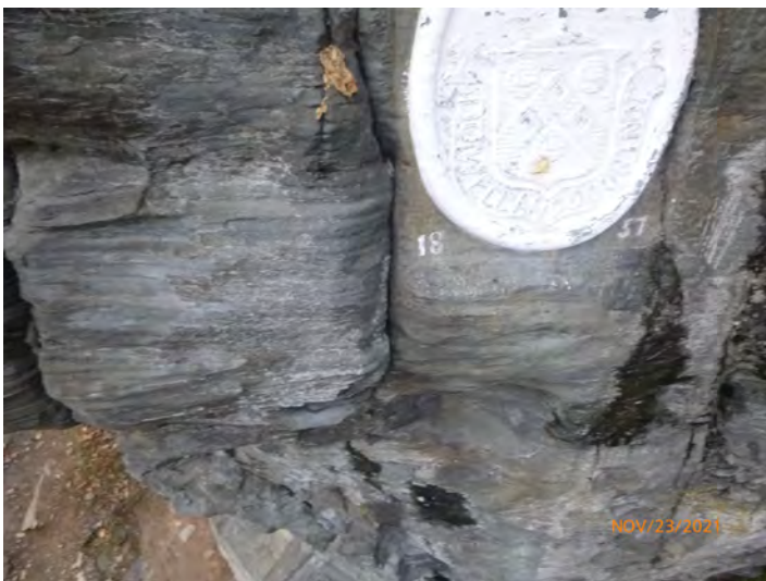
21-18 Stone_Crack Single unit 2021-3
