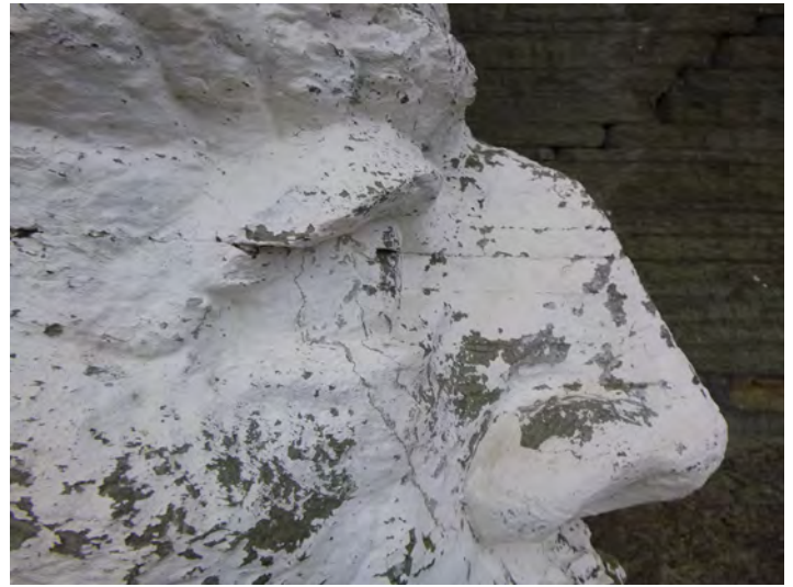
13-23 Stone_Crack Single unit 2021-1
