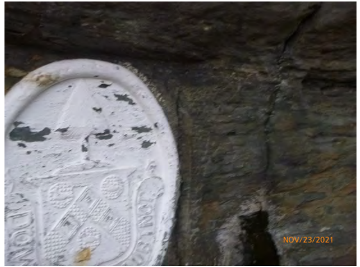
24-17 Stone_Crack Single unit 2021-1
