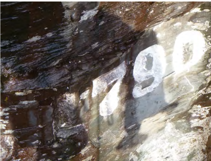
36-14 Stone_Coating Coating Failed 2021-4
