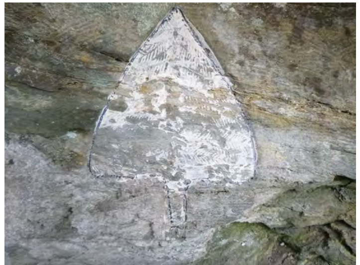
146-20 Stone_Coating Coating Failed 2021-1
