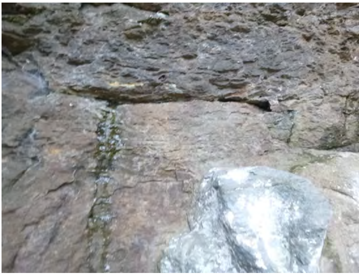
1-15 Stone_Note Photo-water seepage 2021-3
