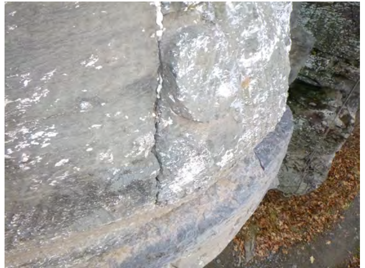
13-20 Stone_Crack Repair failed 2021-1
