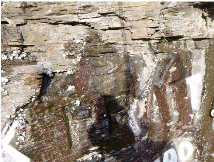
40-17 Stone_Note Photo- Water seepage 2021-1
