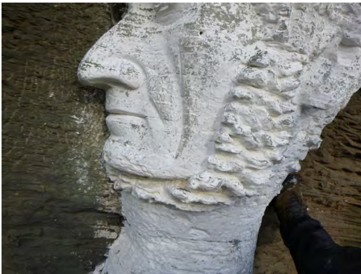
41-27 Stone_Coating Coating Failed 2021-5
