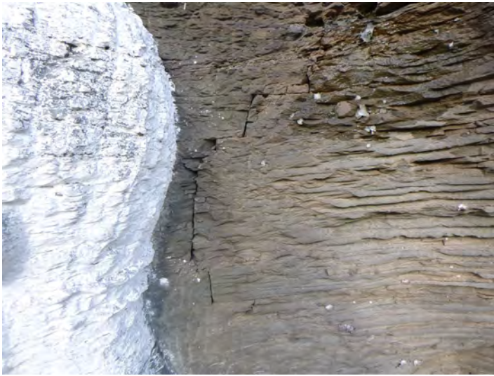
43-26 Stone_Crack Single unit 2021-1
