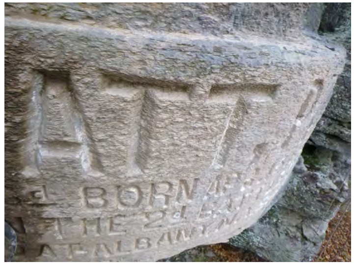
12-18 Stone_Coating Coating Failed 2021-3
