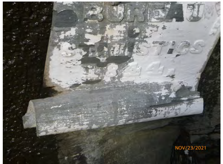
44-9 Stone_Coating Coating Failed 2021-4
