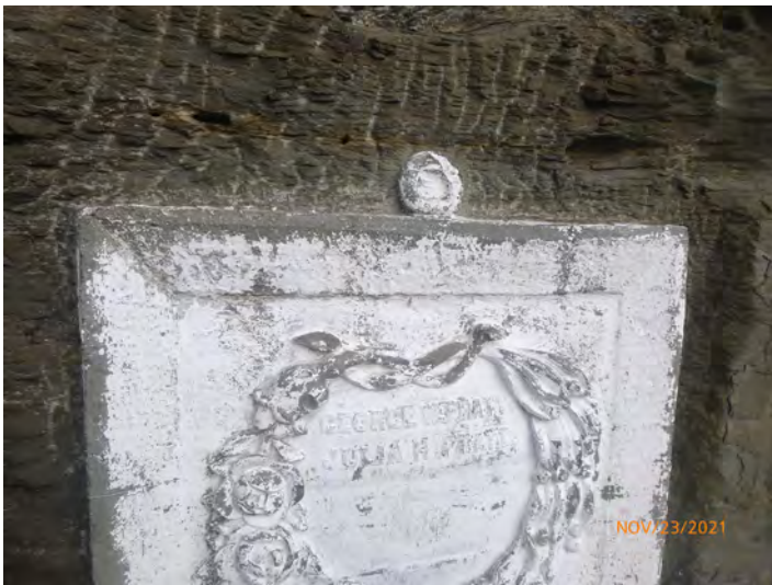
60-14 Stone_Coating Coating Failed 2021-1
