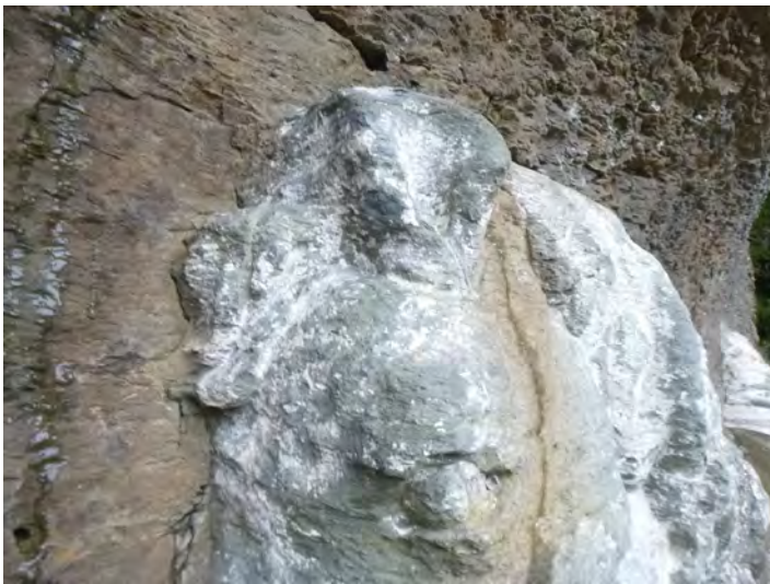
0-12 Stone_Coating Coating Failed 2021-5
