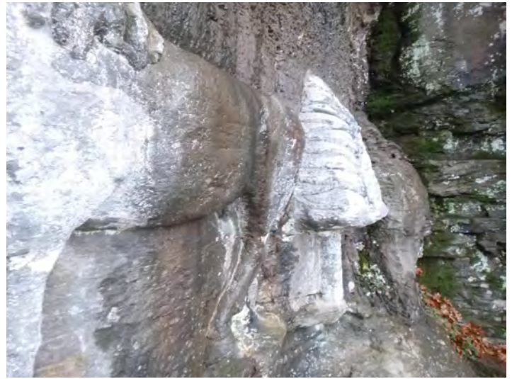
0-13 Stone_Note Photo-water seepage 2021-1
