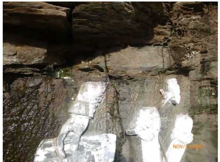
50-8 Stone_Crack Single unit 2021-1
