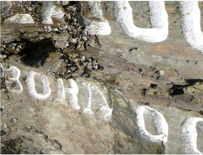
36-14 Stone_Coating Coating Failed 2021-2
