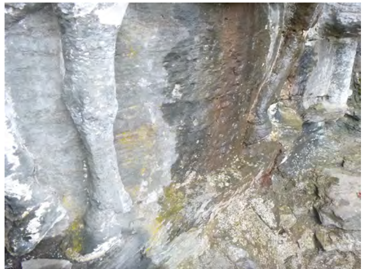
0-12 Stone_Coating Coating Failed 2021-4
