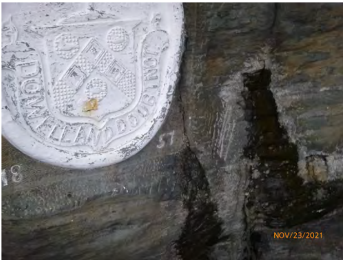
24-17 Stone_Crack Single unit 2021-2
