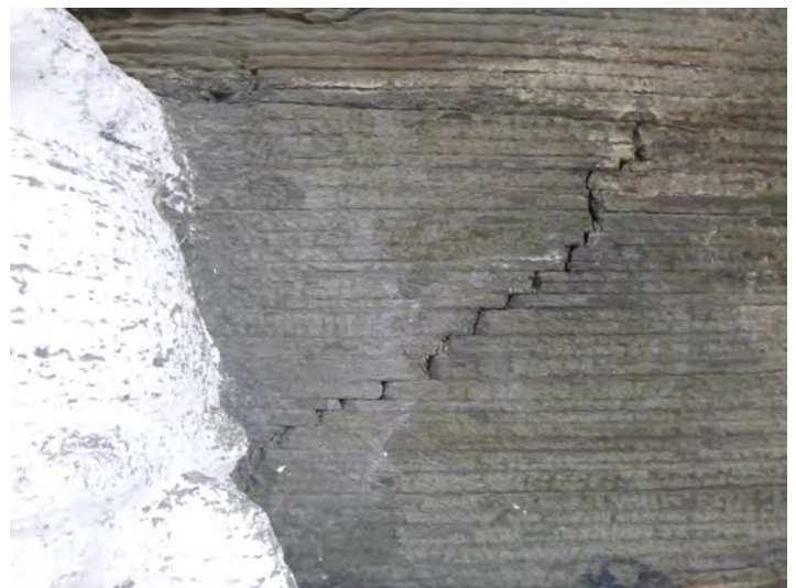
16-23 Stone_Crack Single unit 2021-1
