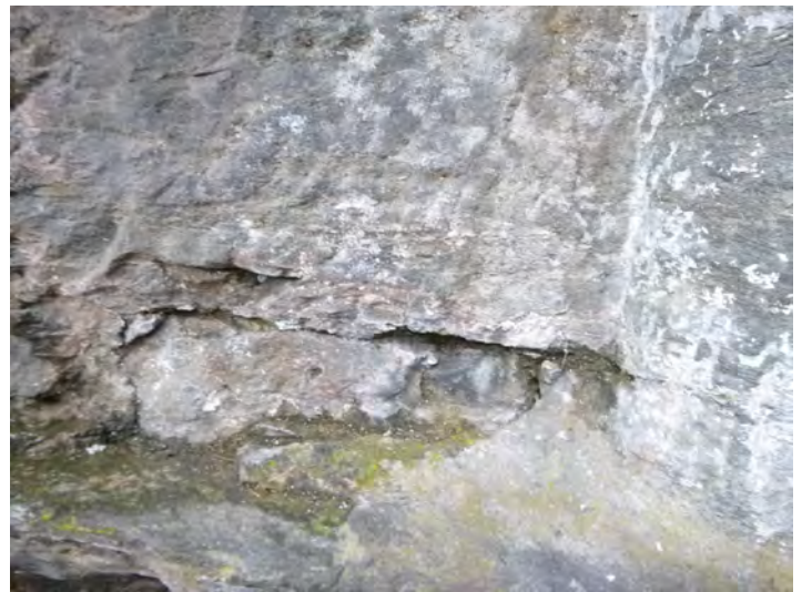
4-11 Stone_Crack System units 2021-1
