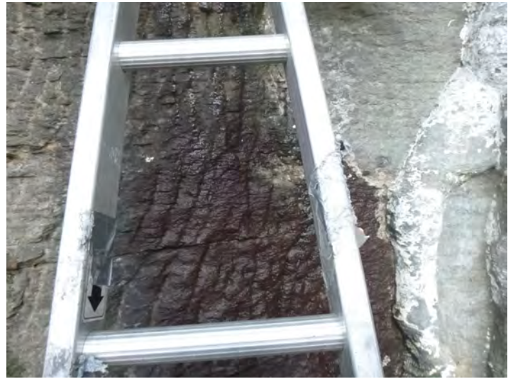
3-13 Stone_Note Photo-water seepage 2021-3
