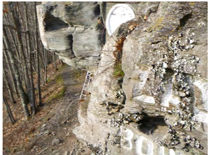
32-17 Stone_Crack Single unit 2021-1
