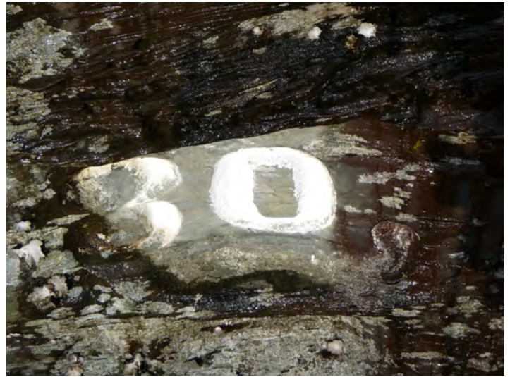
36-14 Stone_Coating Coating Failed 2021-3
