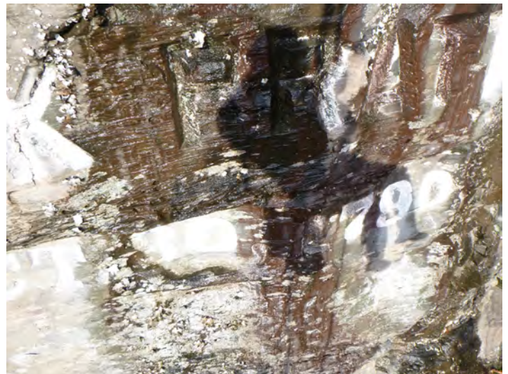
40-17 Stone_Note Photo- Water seepage 2021-2
