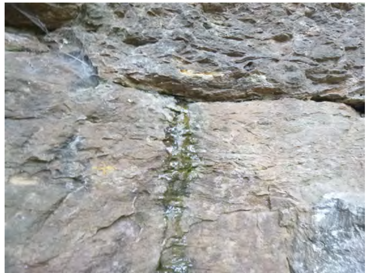
1-15 Stone_Note Photo-water seepage 2021-2
