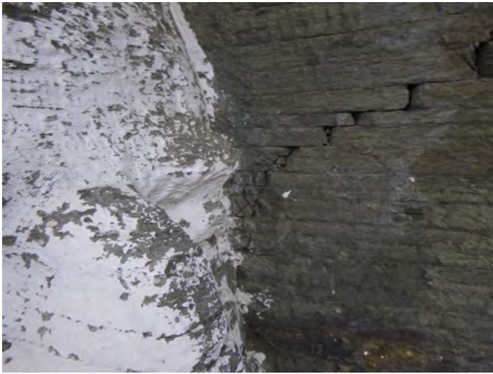
16-23 Stone_Crack Single unit 2021-2
