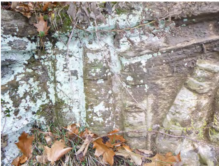
9-20 Stone_Coating Coating Failed 2021-2
