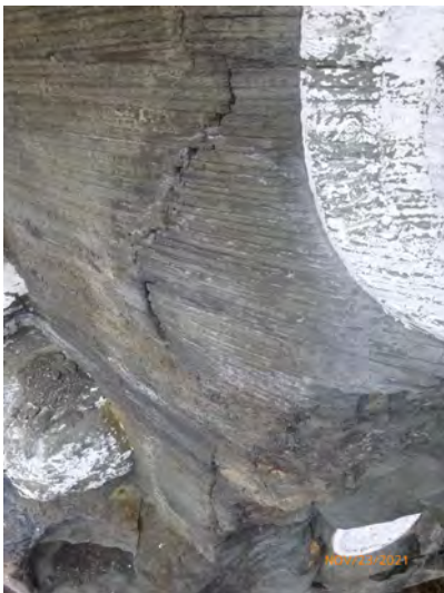
19-22 Stone_Crack Single unit 2021-6
