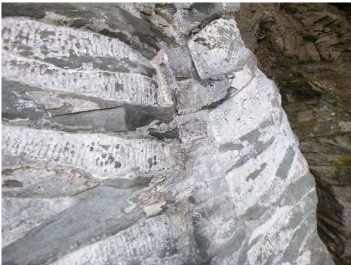
4-13 Stone_Coating Coating Failed 2021-2
