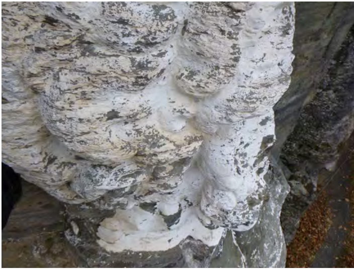
13-23 Stone_Coating Coating Failed 2021-2
