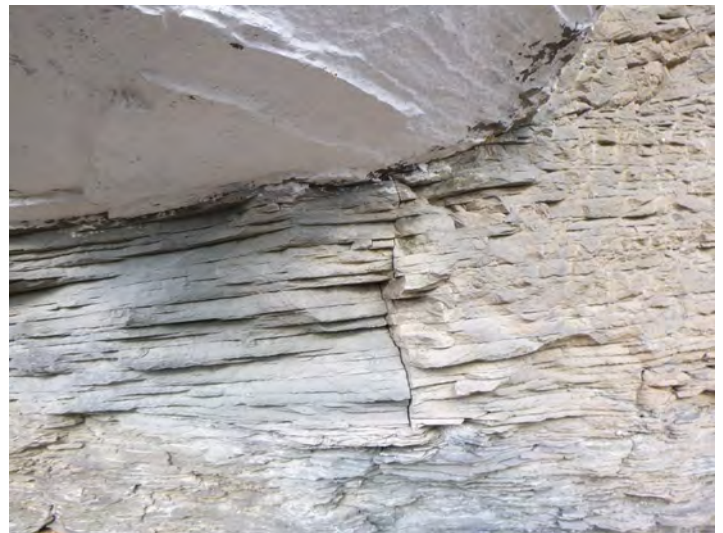
42-22 Stone_Crack Single unit 2021-2
