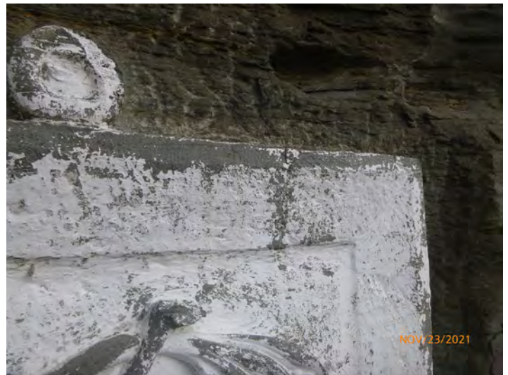
59-15 Stone_Crack Single unit 2021-2
