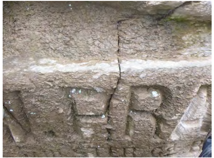
10-18 Stone_Crack Single unit 2021-1
