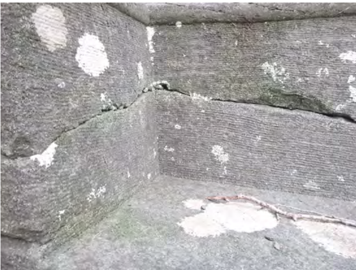
161-26 Stone_Crack System units 2021-4
