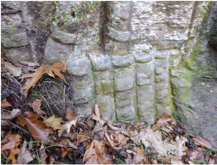
9-20 Stone_Coating Coating Failed 2021-4
