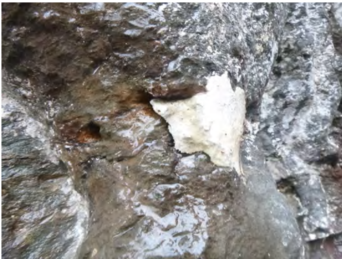
1-12 Stone_Repair Patch Failed 2021-2
