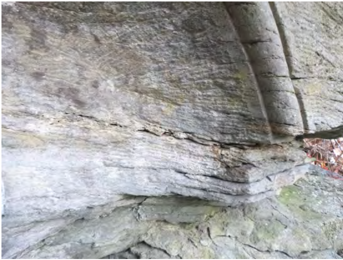
146-20 Stone_Crack System units 2021-1
