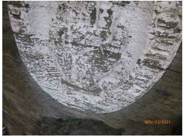
21-22 Stone_Coating Coating Failed 2021-3
