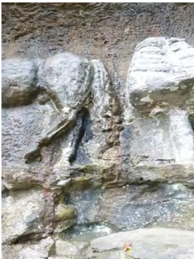
5-11 Stone_Note Photo-water seepage 2021-2
