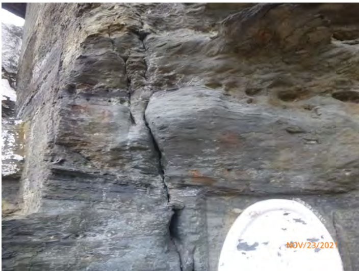
21-18 Stone_Crack Single unit 2021-1
