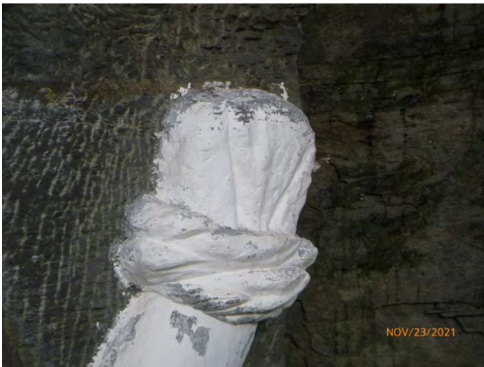
50-8 Stone_Coating Coating Failed 2021-3
