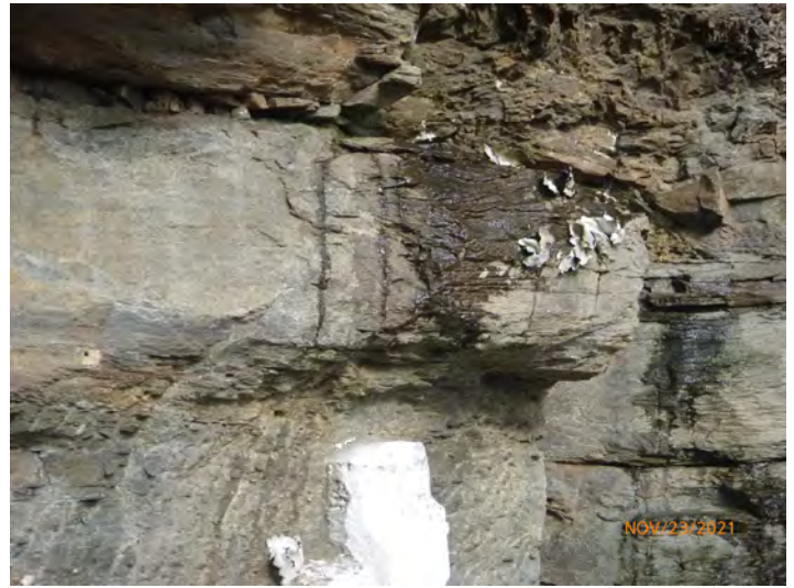
50-12 Stone_Note Photo-water seepage 2021-1
