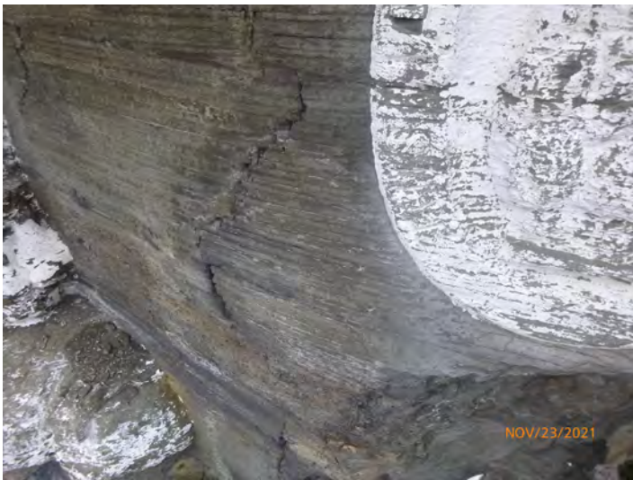
19-22 Stone_Crack Single unit 2021-2
