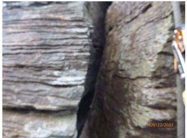
22-34 Stone_Note Photo-fissure above carving 2021-2
