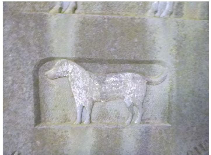
145-27 Stone_Coating Coating Failed 2021-4
