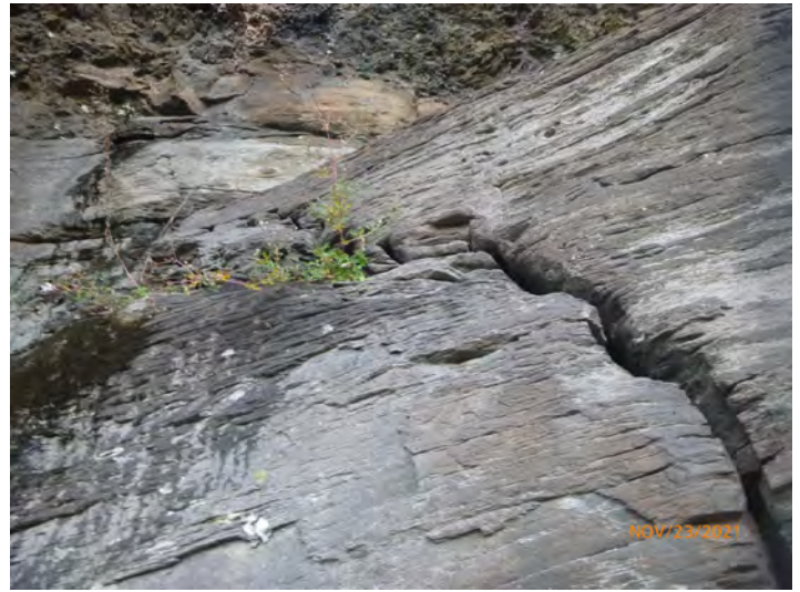
54-15 Stone_Crack Single unit 2021-1
