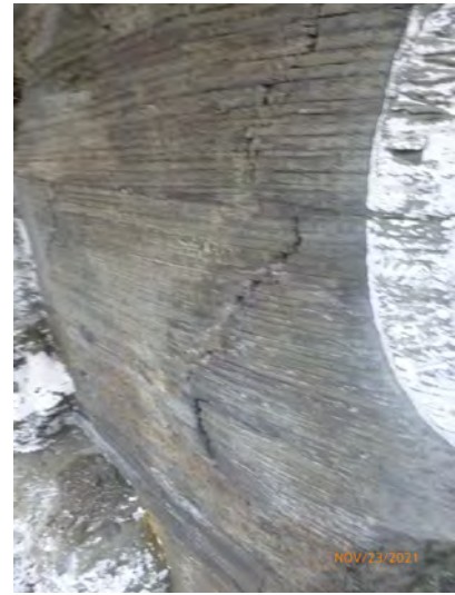
19-22 Stone_Crack Single unit 2021-5
