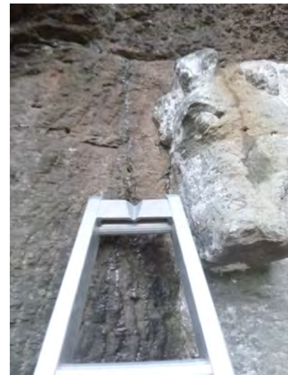
3-13 Stone_Note Photo-water seepage 2021-1
