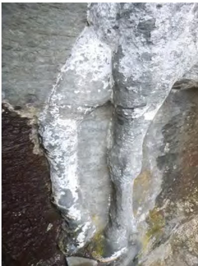
0-12 Stone_Coating Coating Failed 2021-3
