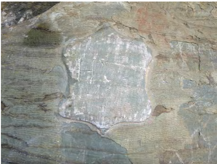
138-15 Stone_Coating Coating Failed 2021-1
