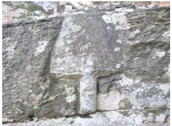
169-26 Stone_Coating Coating Failed 2021-1
