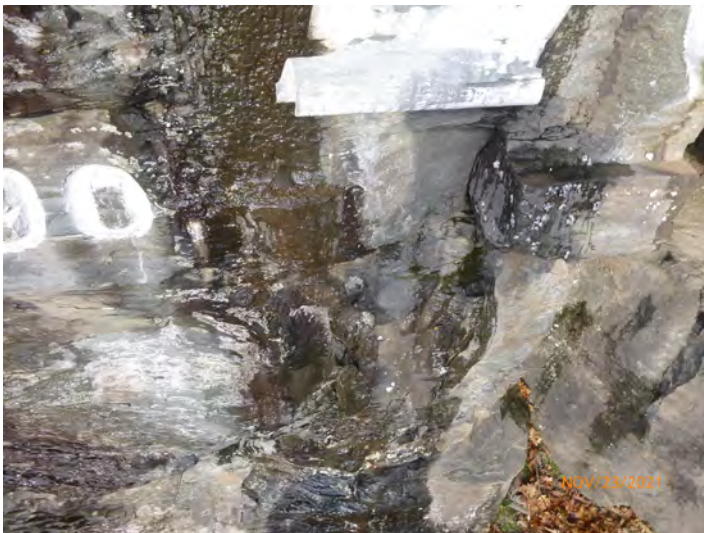
44-12 Stone_Note Photo-water seepage 2021-3
