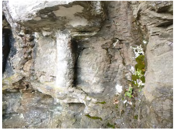
5-11 Stone_Crack System units 2021-1
