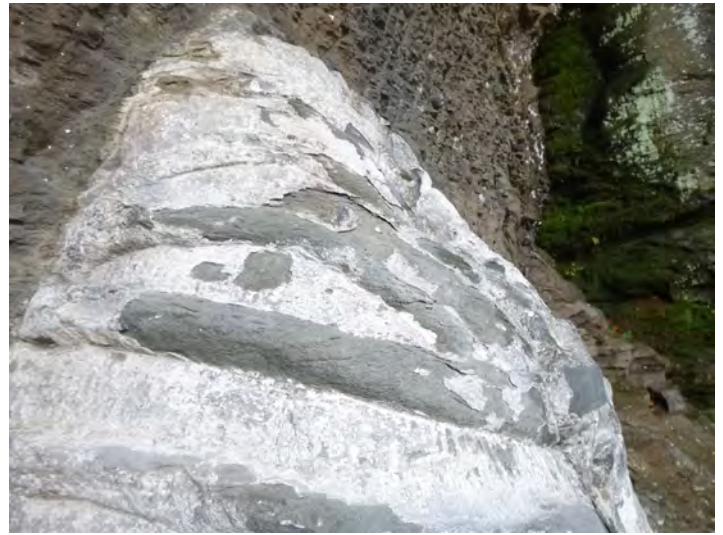
4-13 Stone_Coating Coating Failed 2021-1
