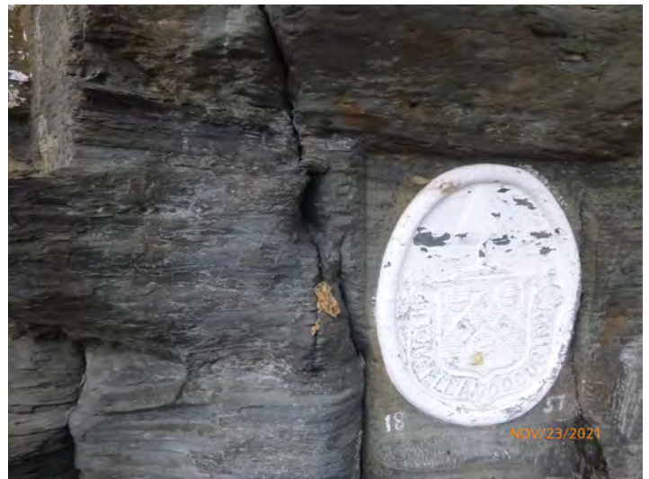
21-18 Stone_Crack Single unit 2021-2
