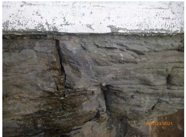
54-15 Stone_Crack Single unit 2021-5
