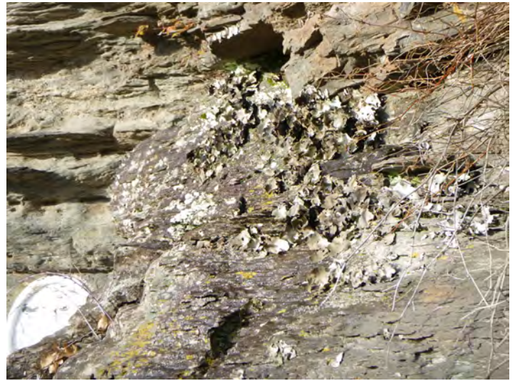
31-18 Stone_Note Photo- Water Seepage 2021-2
