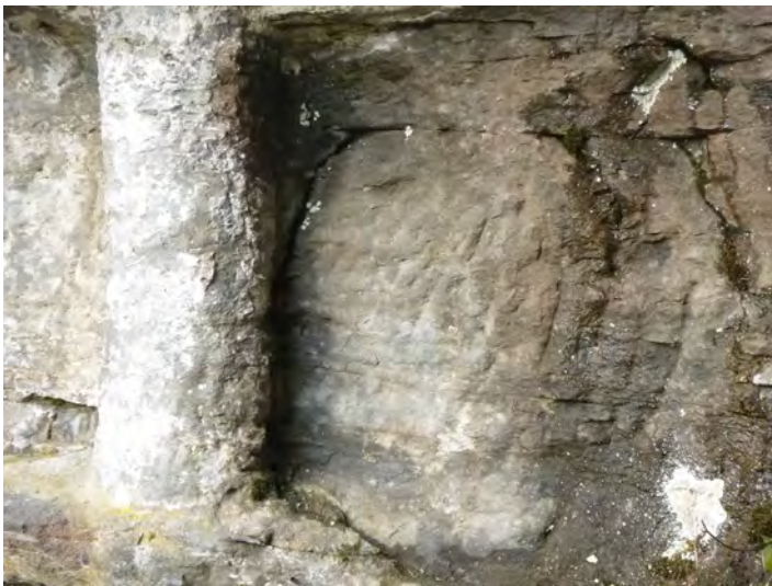
5-11 Stone_Crack System units 2021-2
