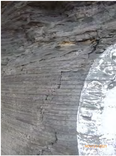
19-22 Stone_Crack Single unit 2021-4
