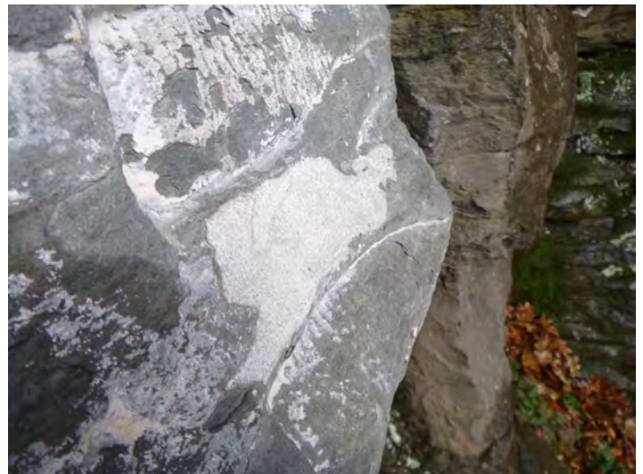
4-13 Stone_Coating Coating Failed 2021-3
