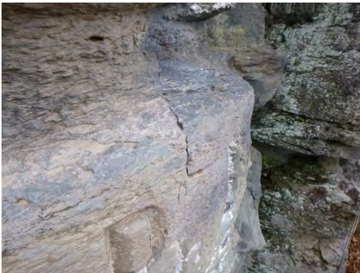
15-19 Stone_Crack Single unit 2021-1
