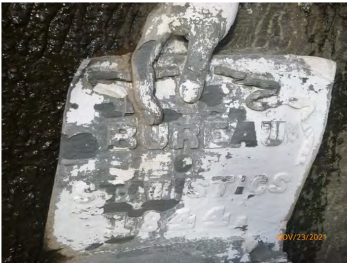
44-9 Stone_Coating Coating Failed 2021-3
