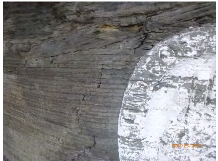
19-22 Stone_Crack Single unit 2021-1
