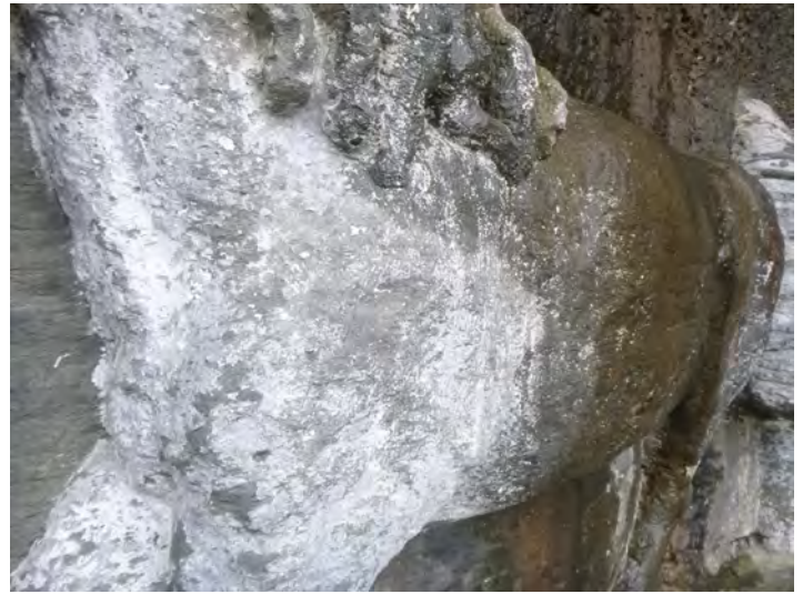
0-12 Stone_Coating Coating Failed 2021-2
