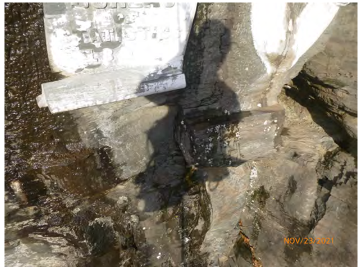
50-8 Stone_Crack Single unit 2021-3
