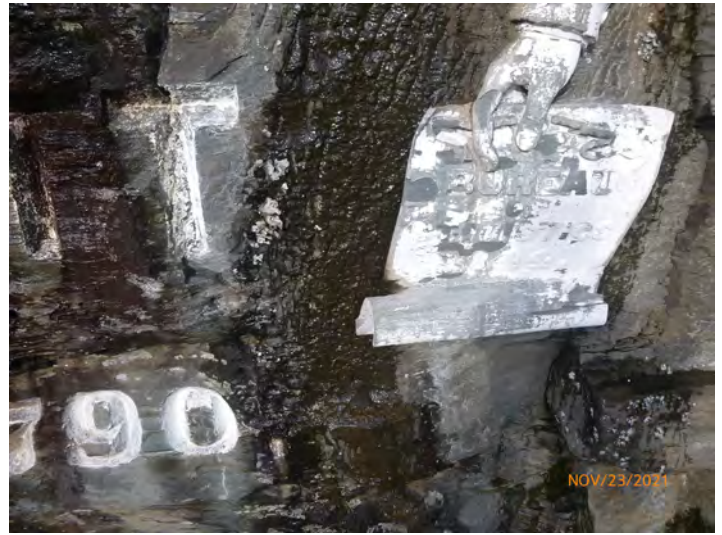
44-12 Stone_Note Photo-water seepage 2021-2
