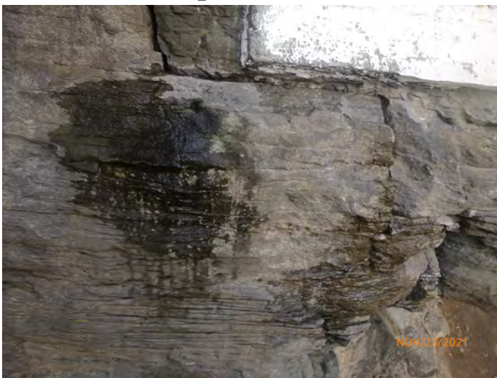
57-10 Stone_Note Photo-water seepage 2021-1
