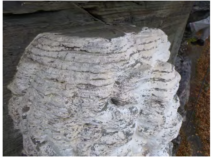
13-23 Stone_Coating Coating Failed 2021-1
