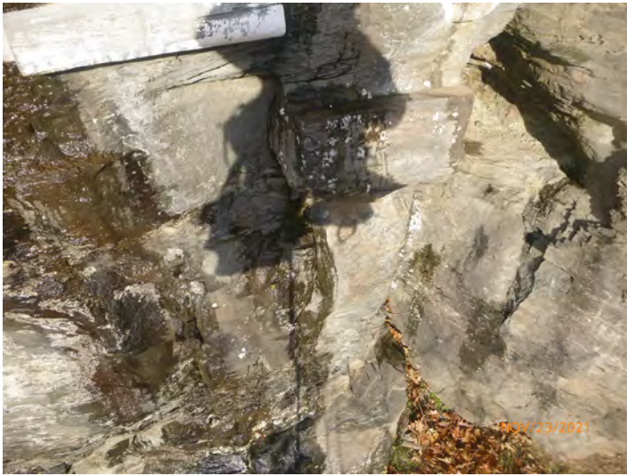
50-8 Stone_Crack Single unit 2021-4
