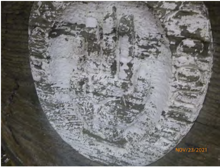
21-22 Stone_Coating Coating Failed 2021-2
