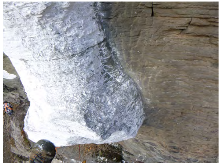
41-27 Stone_Coating Coating Failed 2021-6
