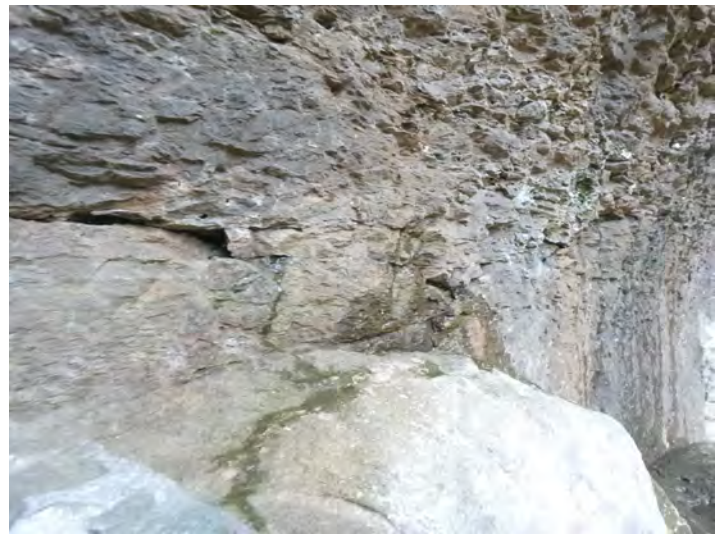
1-15 Stone_Note Photo-water seepage 2021-4
