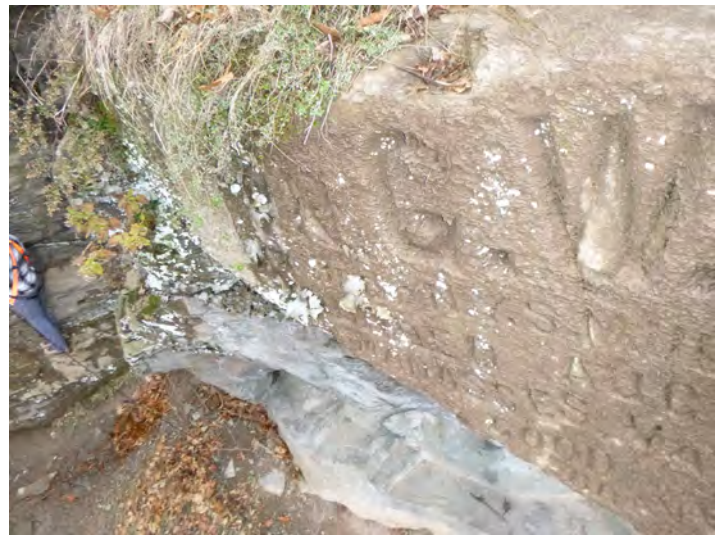
12-18 Stone_Coating Coating Failed 2021-1
