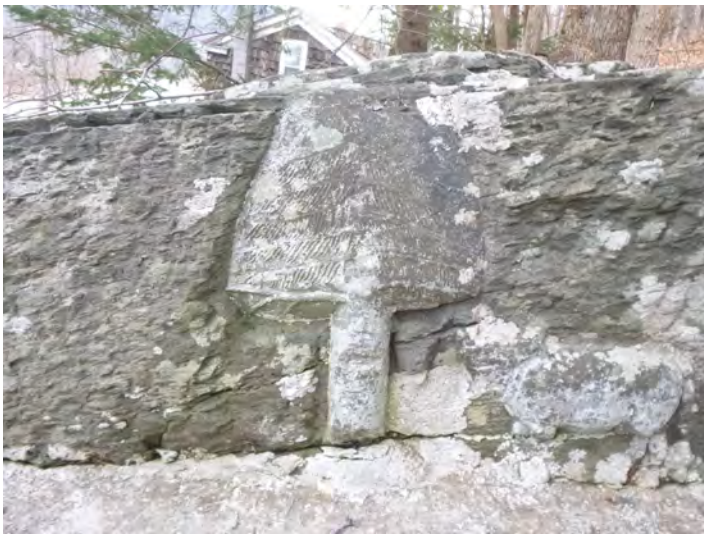
169-26 Stone_Crack System units 2021-1
