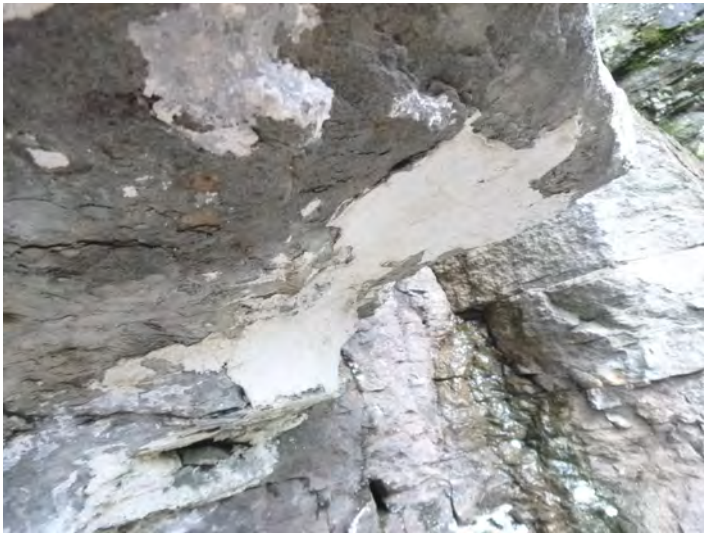
4-13 Stone_Coating Coating Failed 2021-6
