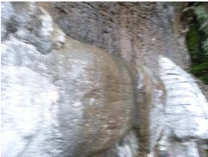
0-13 Stone_Note Photo-water seepage 2021-2
