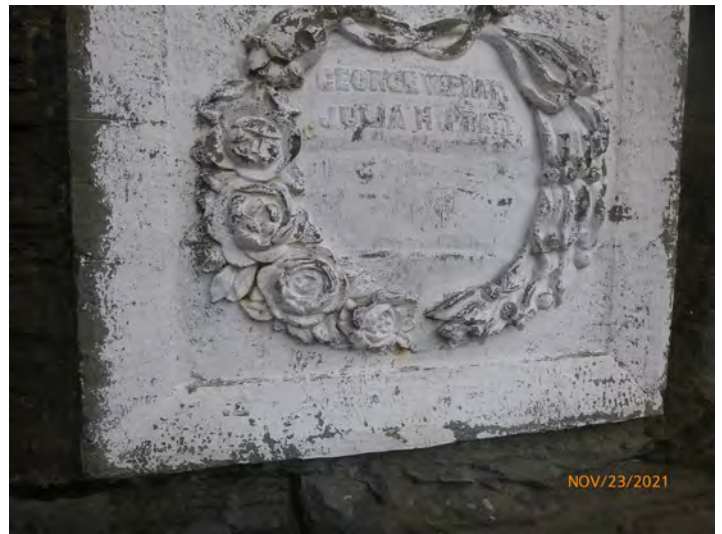
60-14 Stone_Coating Coating Failed 2021-2
