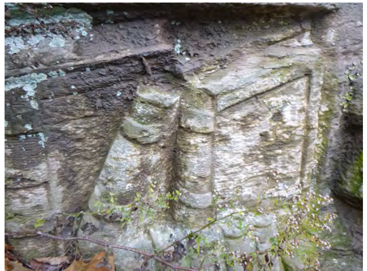
9-20 Stone_Coating Coating Failed 2021-3
