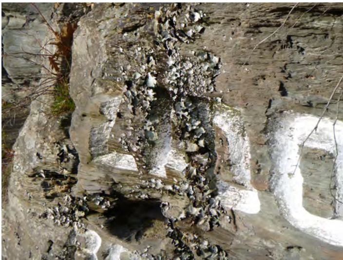
31-18 Stone_Note Photo- Water Seepage 2021-3
