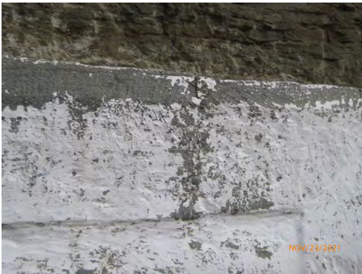
59-15 Stone_Crack Single unit 2021-1
