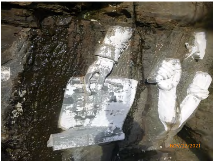
44-9 Stone_Coating Coating Failed 2021-1
