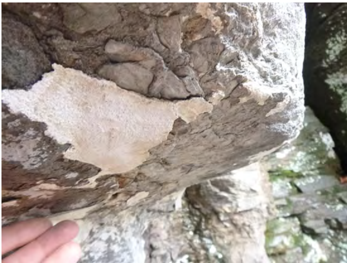
4-13 Stone_Coating Coating Failed 2021-4
