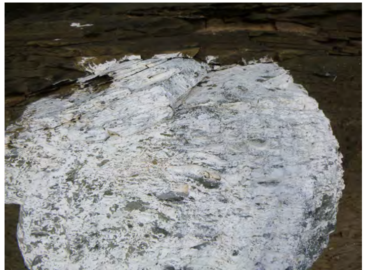
41-27 Stone_Coating Coating Failed 2021-2
