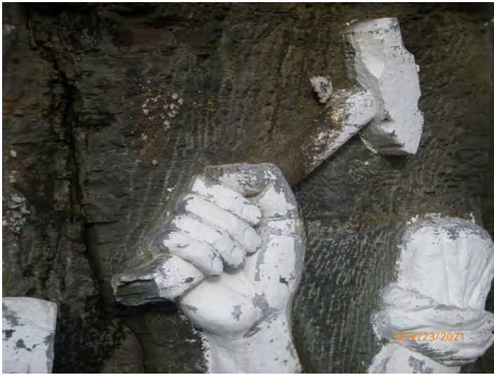
50-8 Stone_Coating Coating Failed 2021-1
