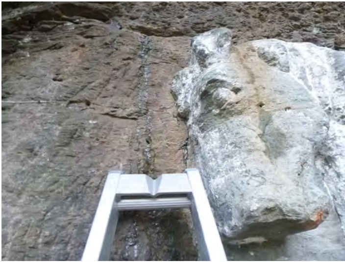
3-13 Stone_Note Photo-water seepage 2021-2
