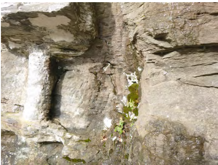
2-12 Stone_Note Photo-water seepage 2021-1
