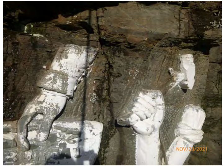
48-13 Stone_Note Photo-water seepage 2021-1
