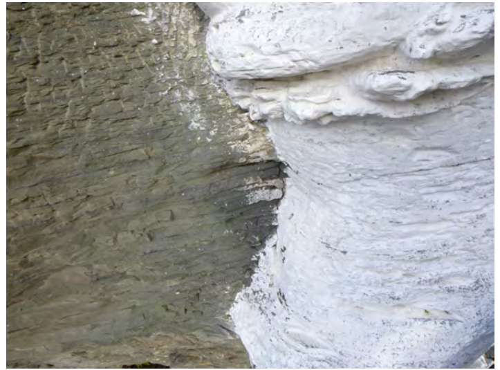
39-24 Stone_Crack Single unit 2021-2
