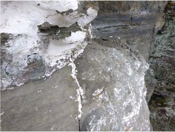
13-20 Stone_Crack Repair failed 2021-2
