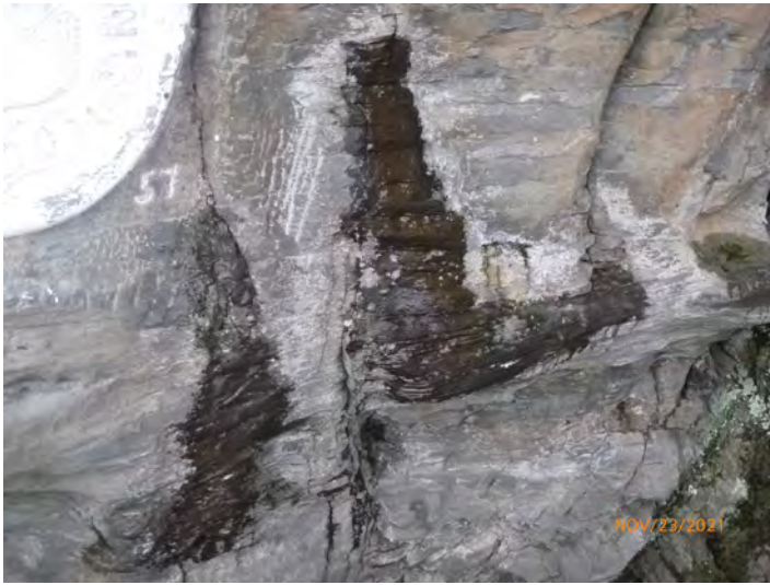
24-14 Stone_Note Photo-water seepage 2021-1
