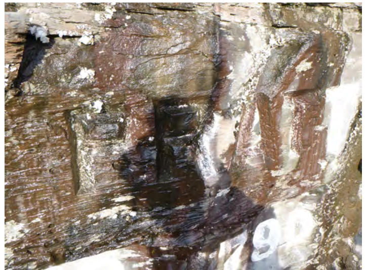
36-14 Stone_Coating Coating Failed 2021-5
