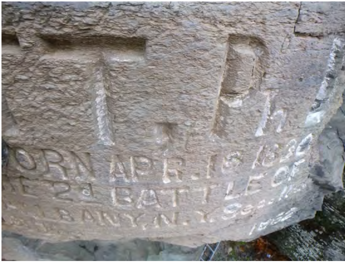
12-18 Stone_Coating Coating Failed 2021-4
