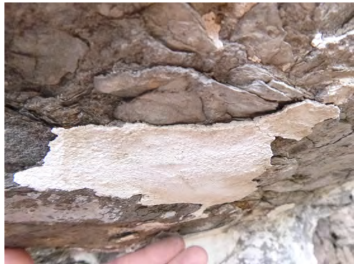
4-13 Stone_Coating Coating Failed 2021-5
