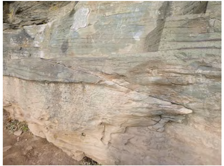
139-14 Stone_Crack System units 2021-3
