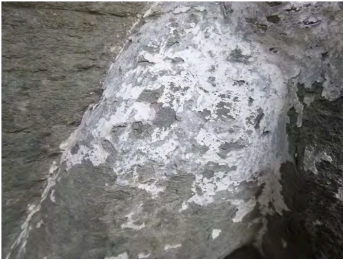
0-12 Stone_Coating Coating Failed 2021-7
