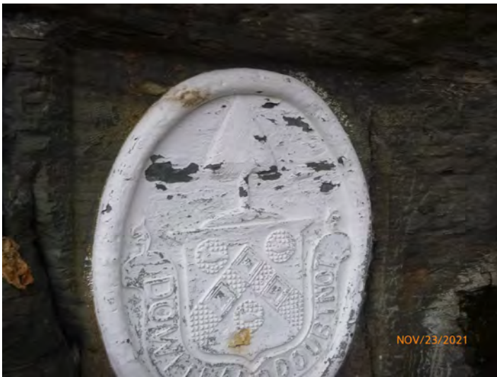
22-16 Stone_Coating Coating Failed 2021-1
