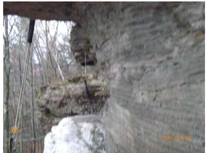
19-27 Stone_Embedment Ferrous Embedment 2021-2
