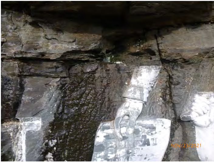
44-12 Stone_Note Photo-water seepage 2021-1
