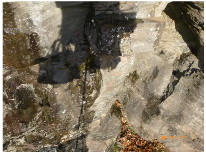
48-13 Stone_Note Photo-water seepage 2021-3
