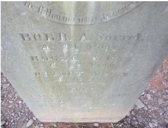
145-27 Stone_Coating Coating Failed 2021-5
